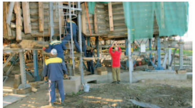
Fig. 10. Dismantling of the VIIth restoration tier elements and fixing of lifted walls on lifting constructions
