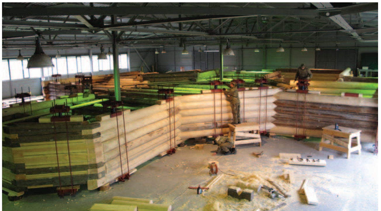
Fig. 12. Installation of metal constructions with jacks for simulation of loadings on the framework
