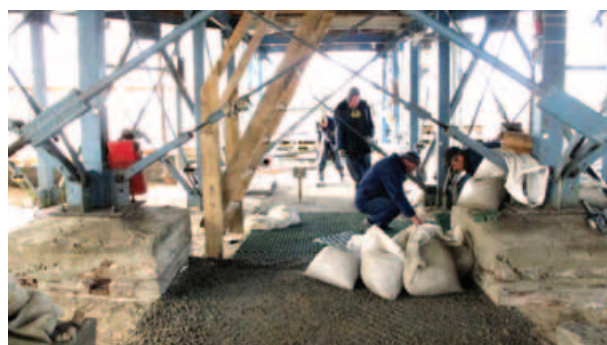
Fig. 8. Ground leveling and laying of polymer mesh in the basement of the Church of the Transfiguration
