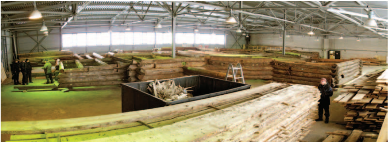
Fig. 12. Framework of the basement (before the restoration) placed in new corrected outline. Beginning of the year 2011
