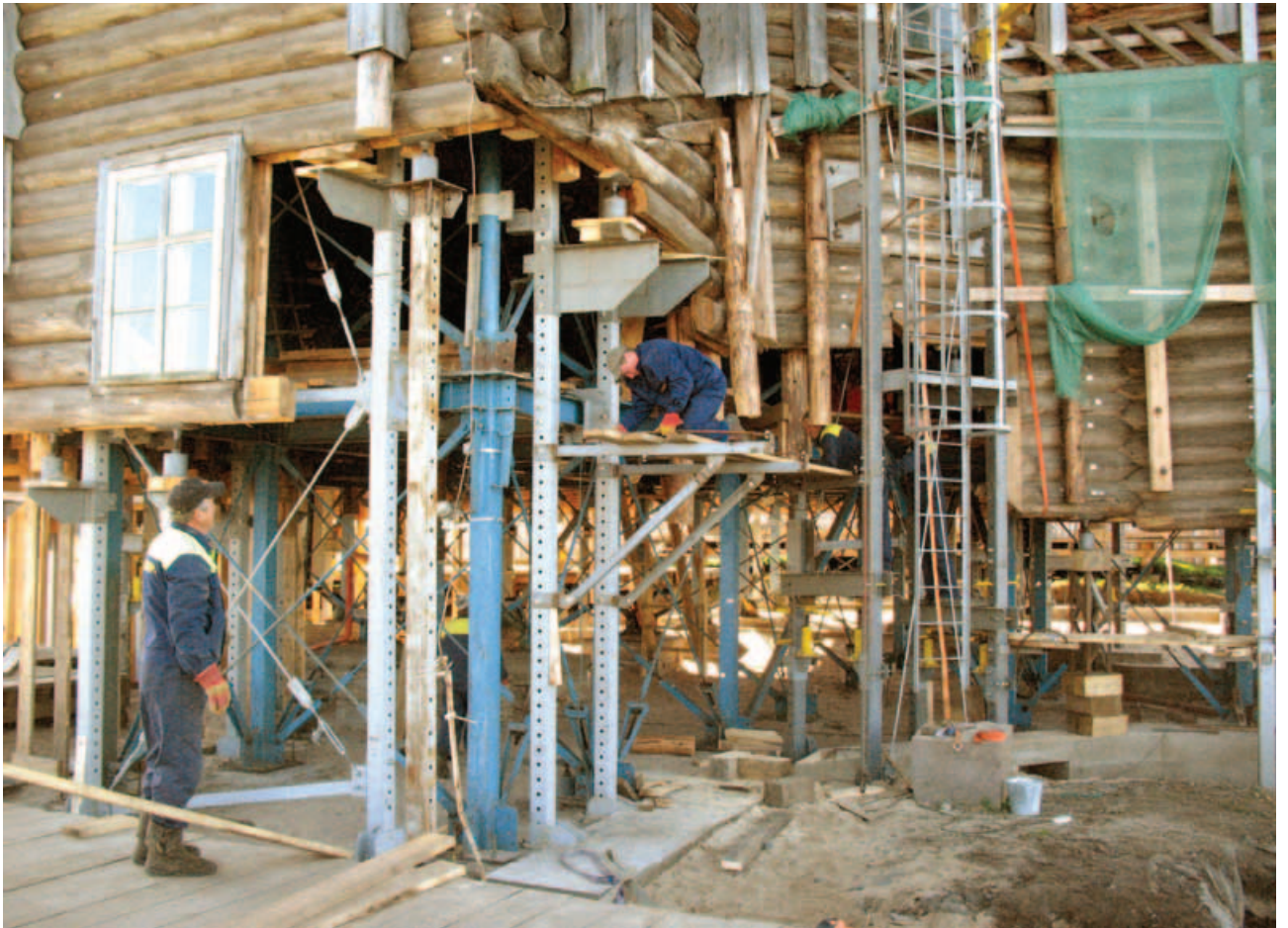
Fig. 5. Dismantling of logs from the Church framework by the use of lifting system.
