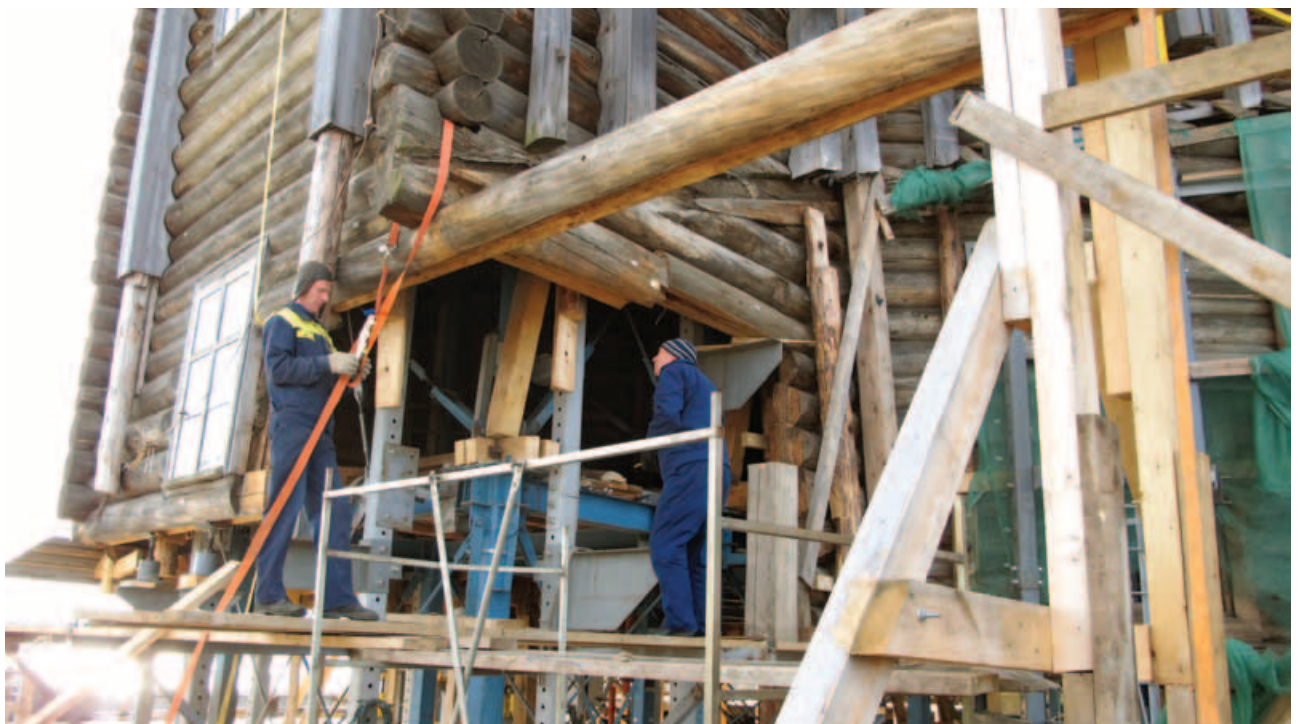
Fig. 6. Logs are dismantling by SKF "Alekon" company fitters. They have been working on the Church since 2004.
