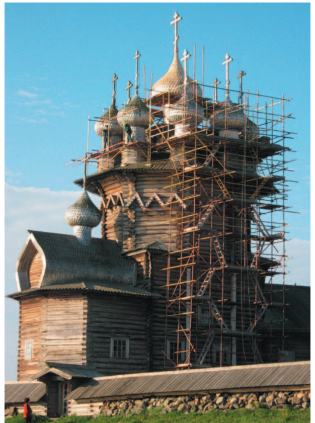
photo 15. The restoration of the domes and roof of the Church of the Intercession in progress.
