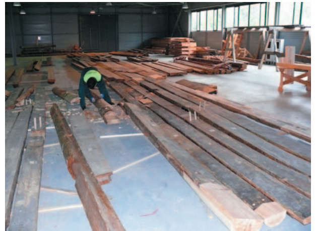
photo 7. General view of the assembly department with the Church floor components being spread and prepared for restoration.
