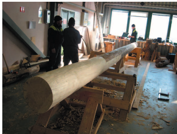
Fig. 16. New wood insertion in a log from the refectory – preservation of a destroyed structural element
