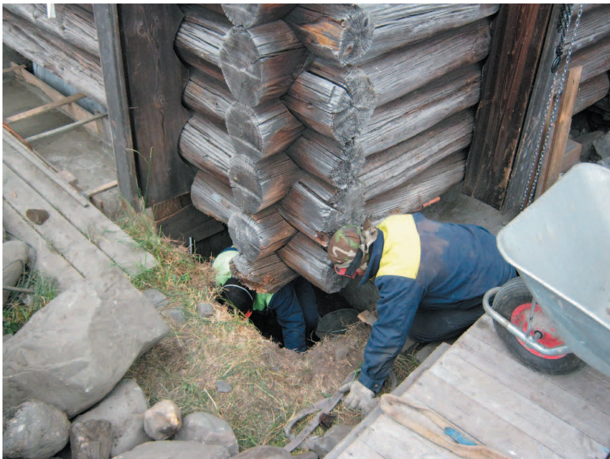
Fig.1. Ditch digging for belt rubble concrete foundation under lifted Church framework. Work of people in narrow conditions.
