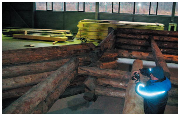
Fig. 31. Installation of beams to historic places – determination of original (XVIII c.) framework geometry
