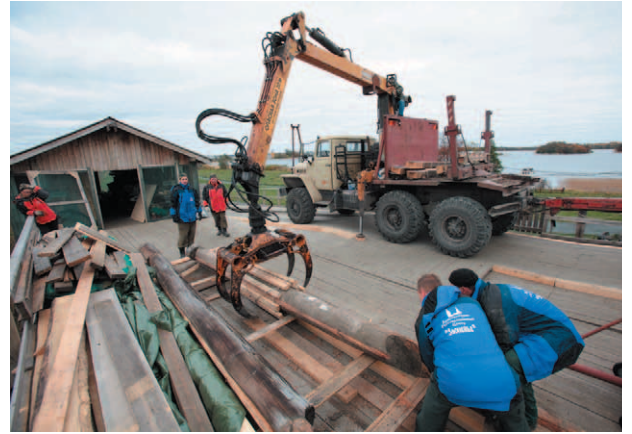
Fig. 26. Loading of logs with the use of special band for transportation to the Restoration Complex
