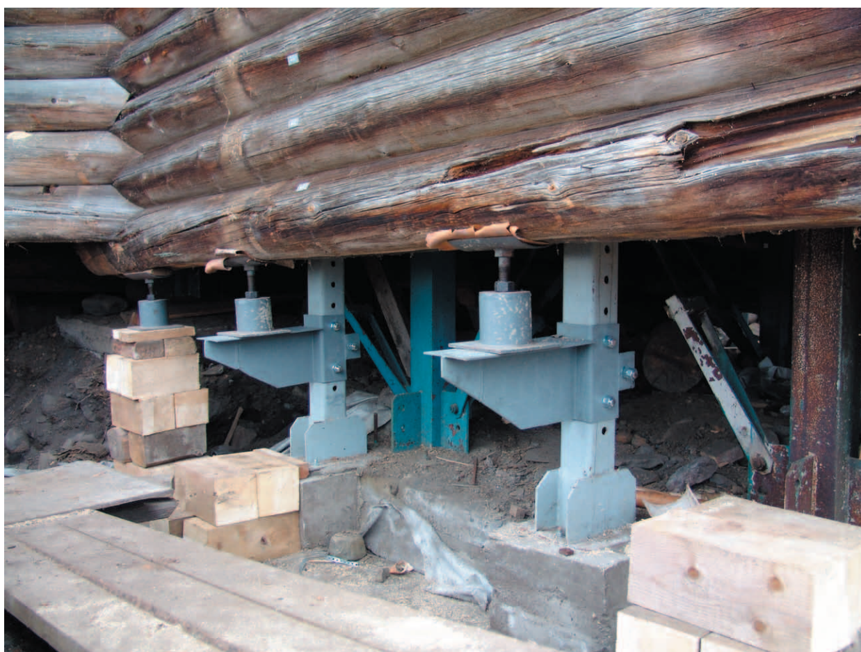
Fig. 4. Initial stage of dismantling. Birch bark is placed between jacks and monument timber
