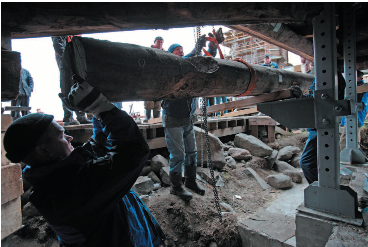
Fig. 13. Final stage of dismantling. Mechanisms of lifting system located along the monument perimeter start to work
