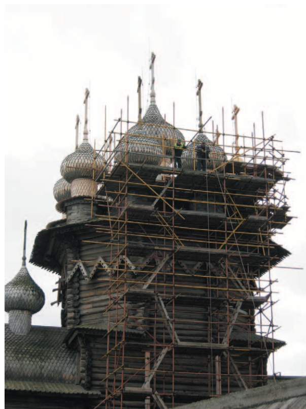
Fig. 38. Dismantling of scaffolding from the northern part of monument and preparation of scaffolding for roof restoration
