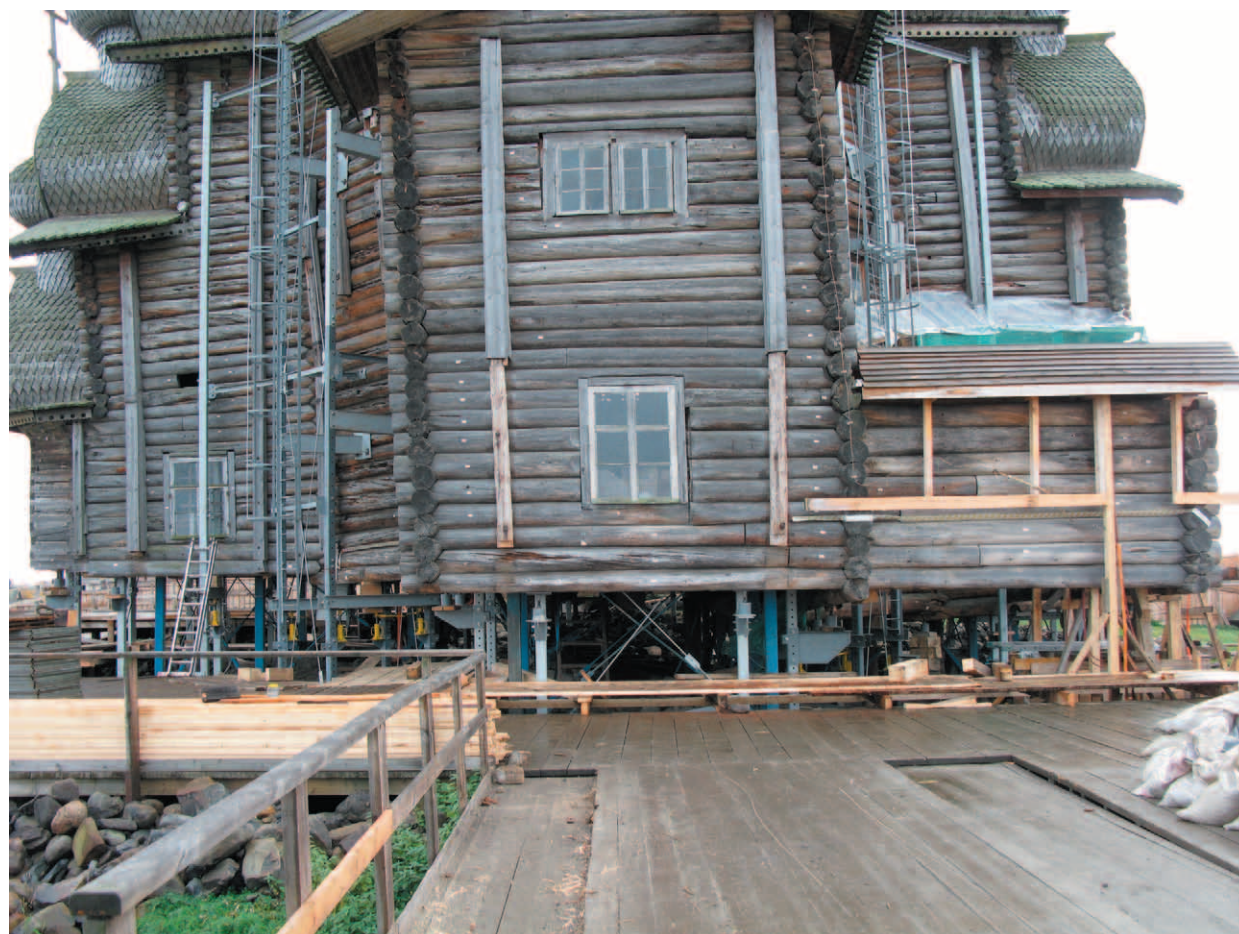
Fig. 18. Final stage of dismantling. General view. 1 timber sets is left along the perimeter
