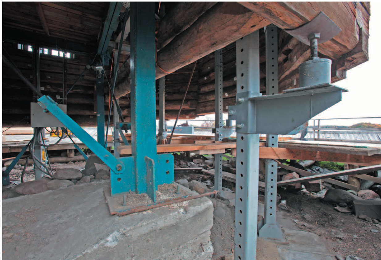
Fig. 12. Sequential dismantling of the Church framework upwards. Regular observations show stable condition of the framework
