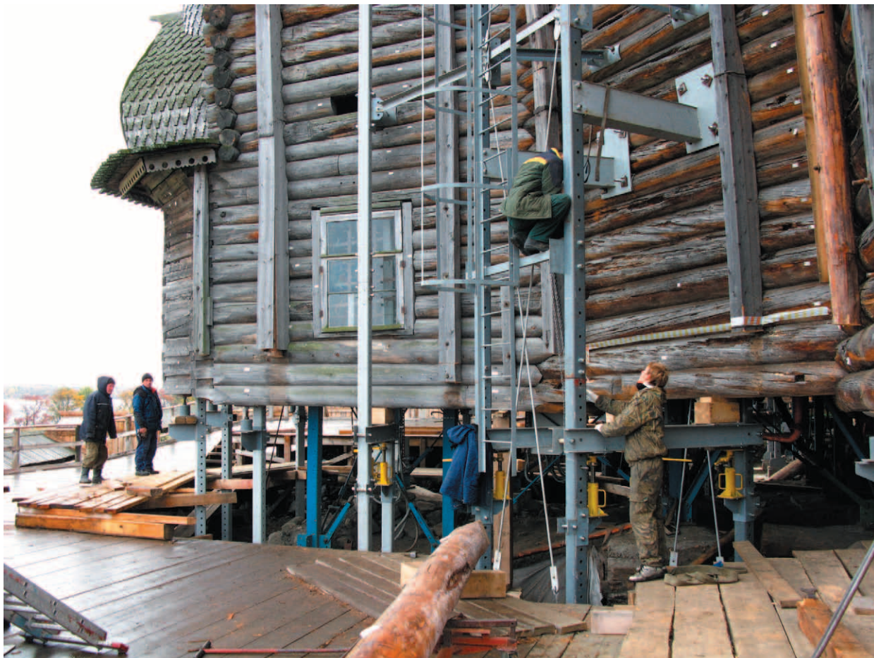
Fig. 17. Final stage of dismantling. General view. 2 timber sets are left along the perimeter
