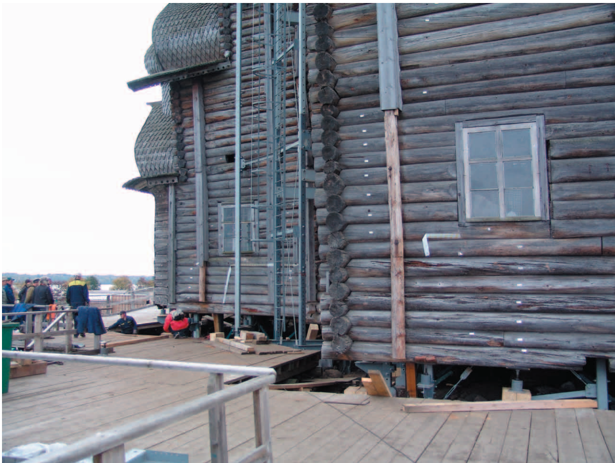
Fig. 5. Initial stage of dismantling. Logs are dismantled along the perimeter in consecutive order
