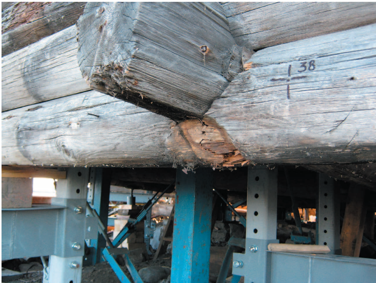
Fig. 11. Invisible defects of logs. The log notch is completely destroyed
