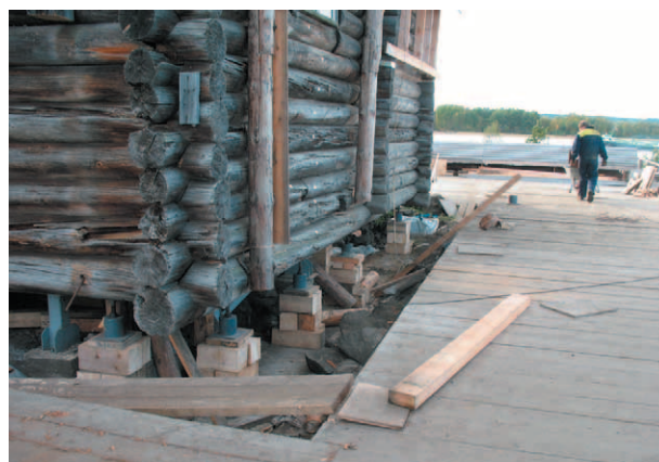
Fig. 22. Initial stage of the dismantling – the Church is supported by jack posts with crawls along the perimeter
