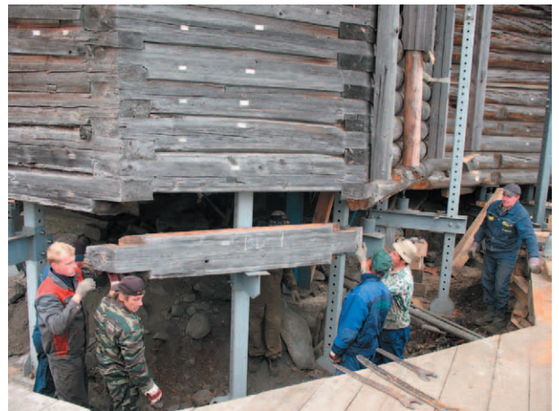
Fig. 24. "Wave" dismantling of the Church framework with the use of lifting system and jacks
