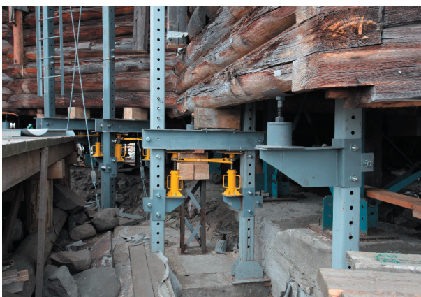
Fig. 12. Movable lifting mechanisms of lifting system: a console, beams and two types of lifting jack
