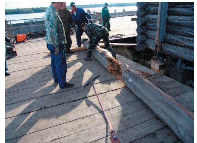
Fig. 28. Inspection during dismantling revealed extremely bad condition of some logs
