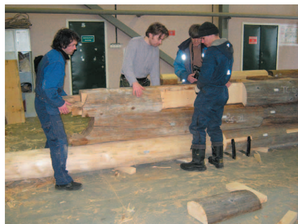
Fig. 19. Restoration of the refectory structural elements with due regard to location of contiguous (upper and lower) elements
